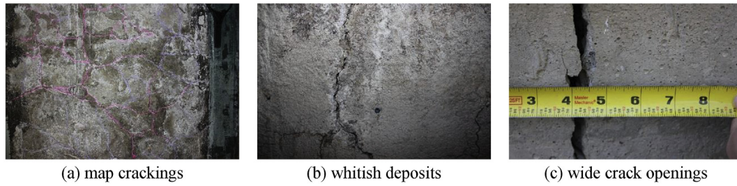
Fig. 1. Common symptoms of deteriorated concrete foundation.
