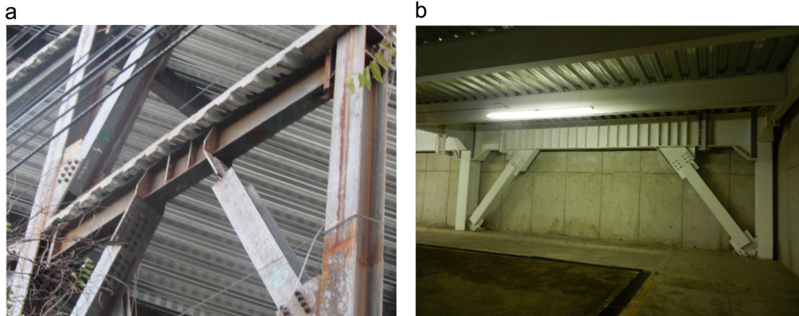
Fig. 1. Examples of the use of eccentric braced frames in buildings: a) short link, b) long link.
