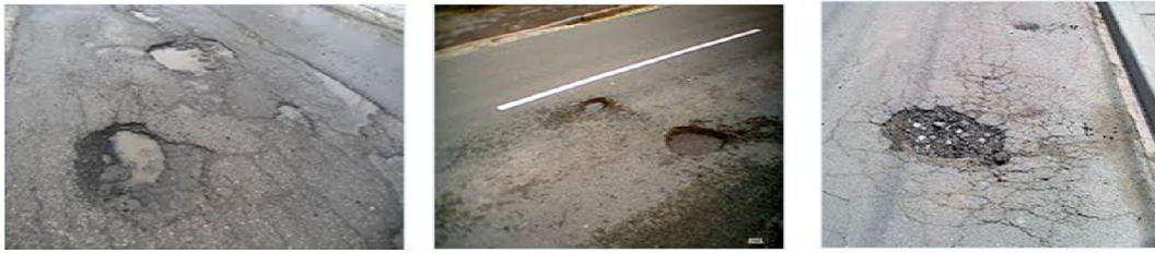
Fig. 1. Different appearances of potholes in the pavement surface.
