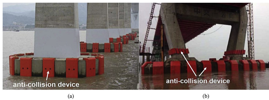
Fig. 1. Application of the orthogonal lattice-web reinforced composite sandwich panels as anti-collision devices: (a) Langqi Min River Bridge and (b) Oubei Bridge.
