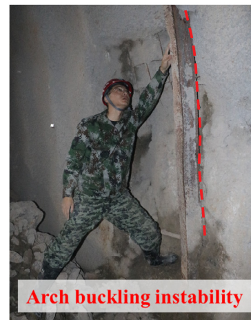
(b) Arch buckling instability
