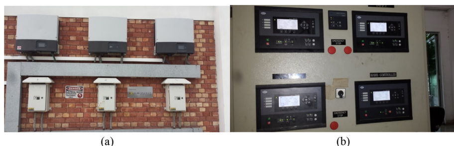
Fig. 1. Grid-tie inverter and display of the diesel generator output at the University of Lahore.
