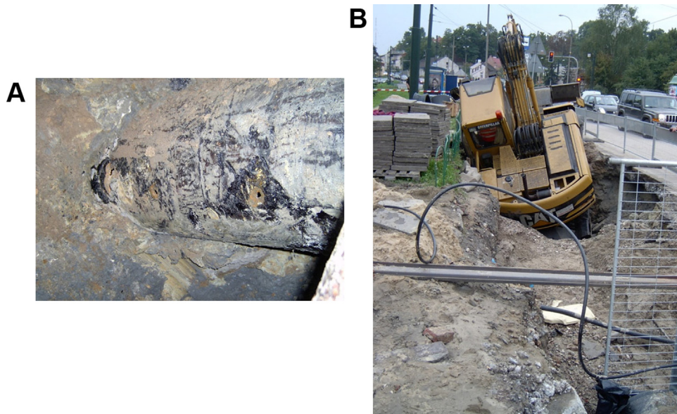
Fig. 1. Local corrosion of a DN300 pipeline.
