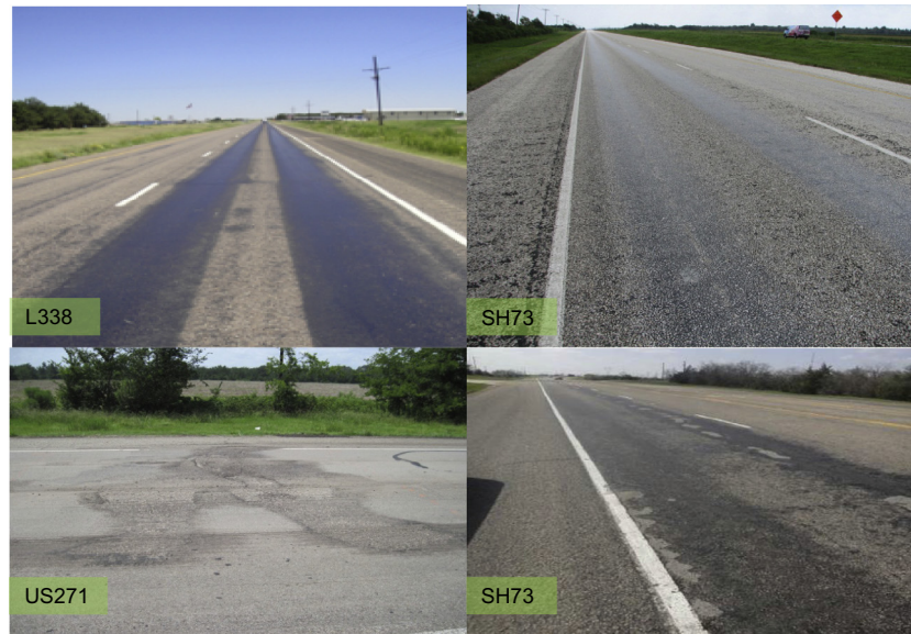
Fig. 1. Candidate pavements for Very Thin Overlays (VTO) with bleeding and raveling surfaces.
