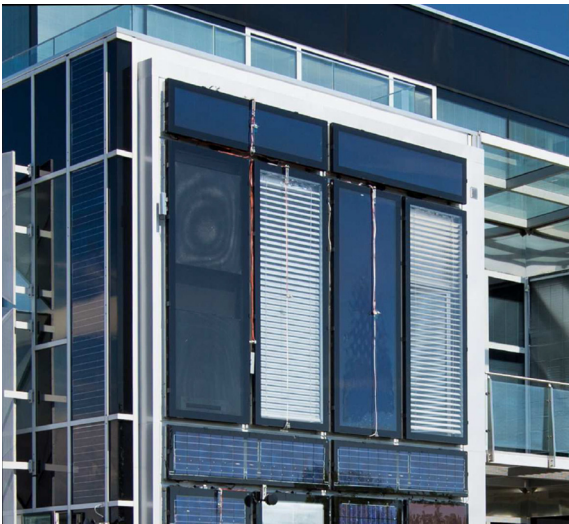
Fig. 1. Prototype installation of a solar thermal facade element developed in MPPF – Multifunctional Plug & Play Facade [5]. Overheating of the interior wall behind the solar thermal elements was observed when the collector was in stagnation.
