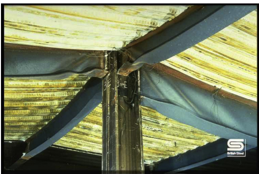
Fig. 1. Shear buckling phenomenon in Cardington fire test [5].
