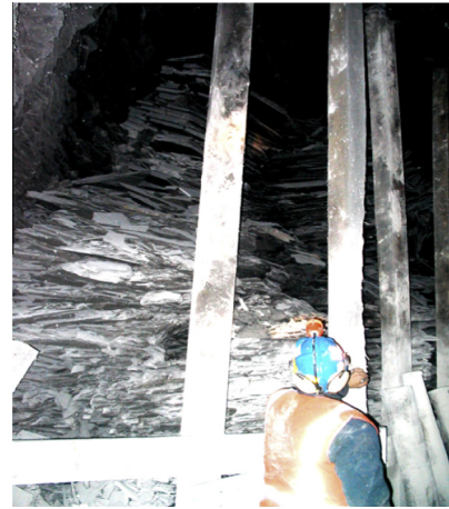
Fig. 2. Large roof fall at Mine A showing laminated nature of the silty shale roof rocks and steep-sided collapse cavity.
