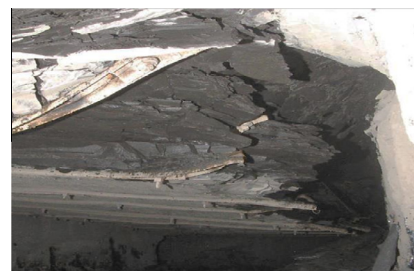
Fig. 3. Severe cutter formation and roof cantilevering at Mine B.
