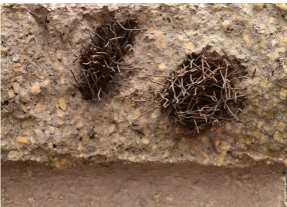
Fig. 1. Fibre balling in a concrete element.
