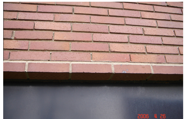
Fig. 3. Repointed bed joint that cracked due to further corrosion of the reinforcement.
