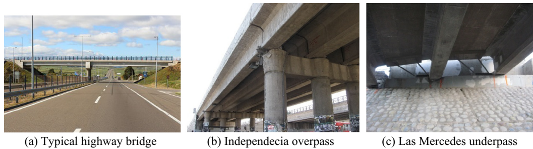
Fig. 1. Typical highway bridges in Chile and observed damage after the 2010 Maule earthquake.
