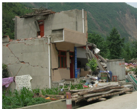
(a) Collapsed masonry building near Beichuan County, having no reinforced concrete columns and beams
