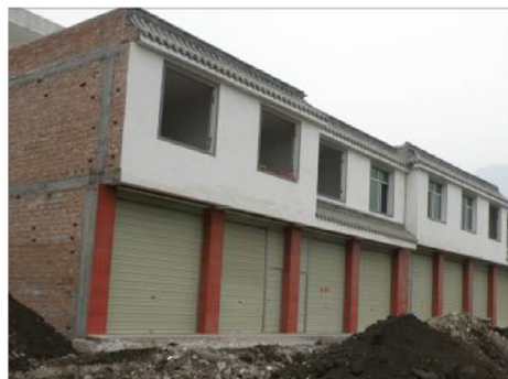
(d) Masonry building at Pengzhou, Bailu Town in good condition, having reinforced concrete columns and beams
