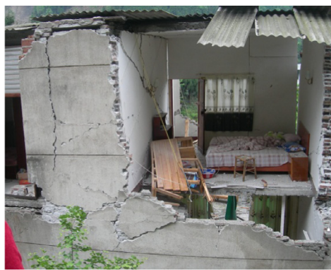
(b) Severely damaged masonry building with collapsed precast slab, having no reinforced concrete columns and beams
