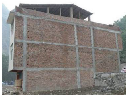
(c) Masonry building near Pingtong Town in good condition, having reinforced concrete columns and beams
