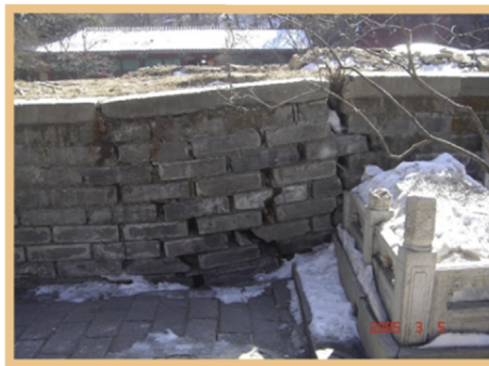
(a) Cracked brick wall.
