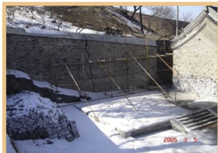
(c) Leaned retaining wall.
