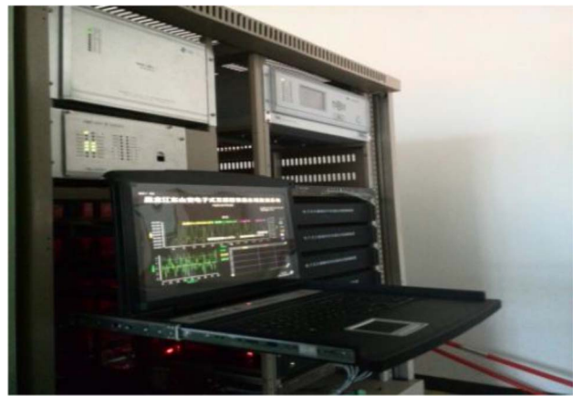
Fig. 4. Indoor field operating error test system devices.
