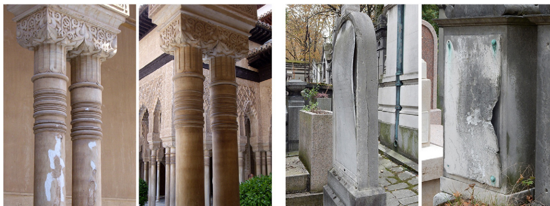
Fig. 1. Examples of thermally induced degradation of marble. Left: Marble columns in the Courtyard of the Lions in the Alhambra of Granada (Spain, XIV century) exhibit severe granular disintegration in the side directly exposed to solar radiation, while in the opposite sheltered side the same columns are substantially well preserved. Right: Thin slabs used as gravestones in the Père Lachaise Cemetery in Paris (France, XIX century) exhibit dramatic bowing and deformation.
