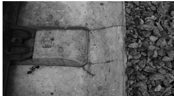
Fig1. Cracks at the experimental stage Sablino – Tosno.
