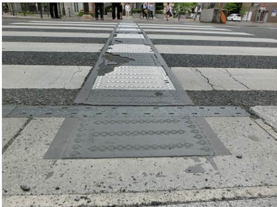
Fig. 1. Example of erosion of protrusions on crosswalk.
