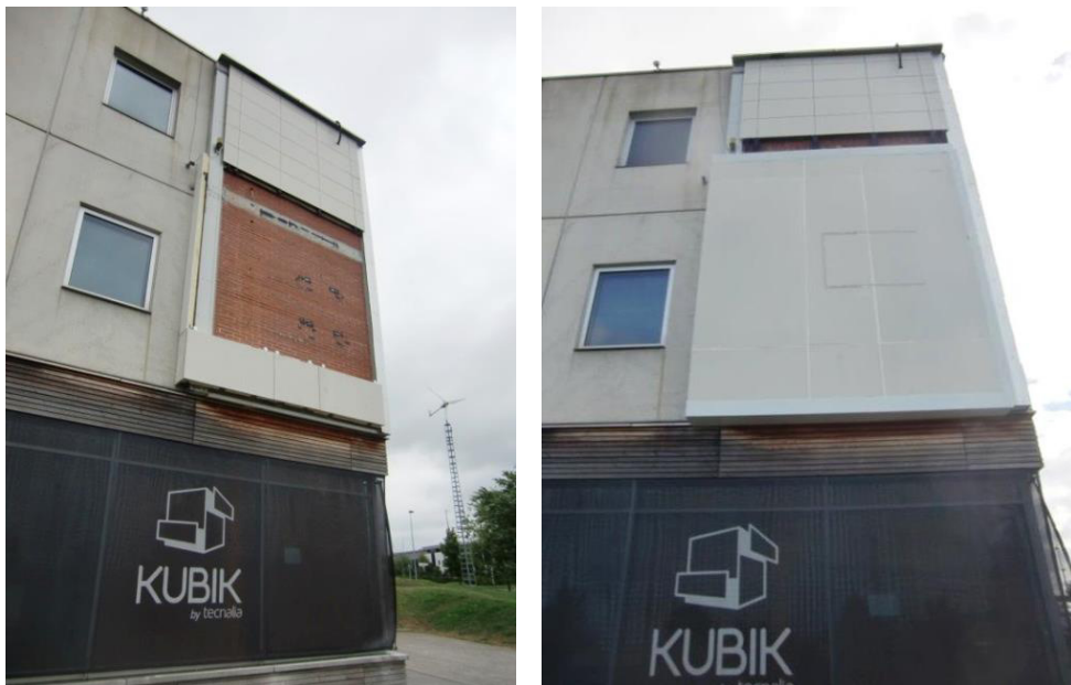
Fig. 1. Test area at first floor of west-facing façade in KUBIK facility: (a) original brick wall before installation; (b) ETIXc prototype installed.
