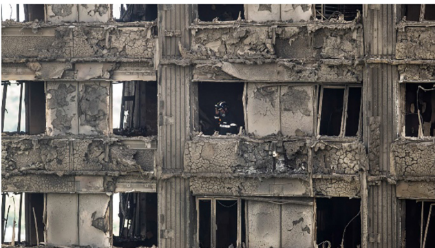
Fig. 2. Facade of the Grenfell tower in the aftermath of the fire.
