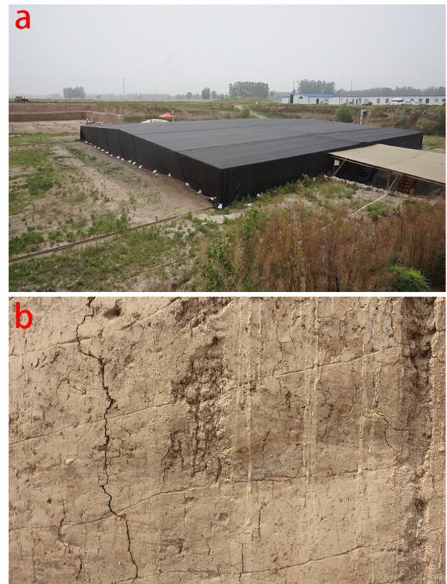
Fig. 1. The earthen site to be protected, a: overall view of mausoleum of the king of Dingtao; b: typical cracking disease on the tomb wall.
