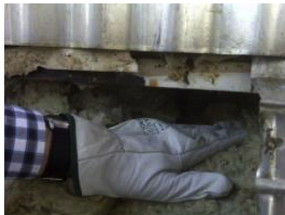
Fig. 3. Lack of insulation material in the storage tanks.
