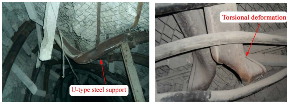
Fig. 1. U-type steel support distortion deformation in a 1200-m-deep roadway in the Huafeng coal mine.
