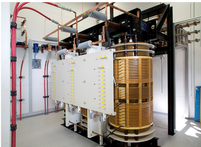
Fig. 2. Three-phase transformer with a switch panel for the fine-adjustment of the test-voltage.
