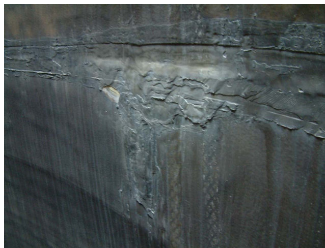
Fig. 1. The coating protecting the area of joining two chimney segments.
