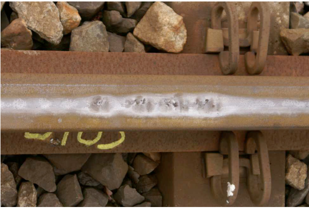
Fig 1: Example of severe squats on a rail
