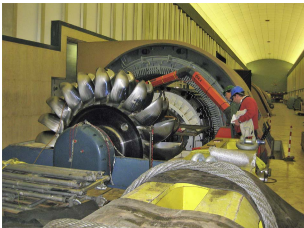
Fig. 1. Pelton turbine open for inspection. The turbine runner and the electrical generator can be seen.
