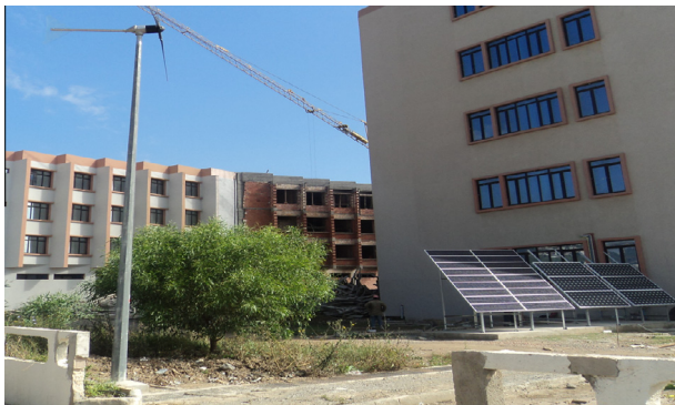
Fig. 1. Installed hybrid wind-photovoltaic system.
