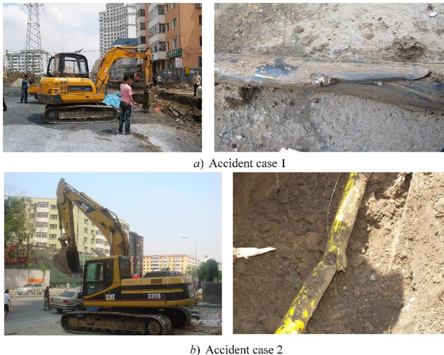
Fig. 1. Urban PE gas pipes accidents caused by mechanical excavator during pavement construction.
