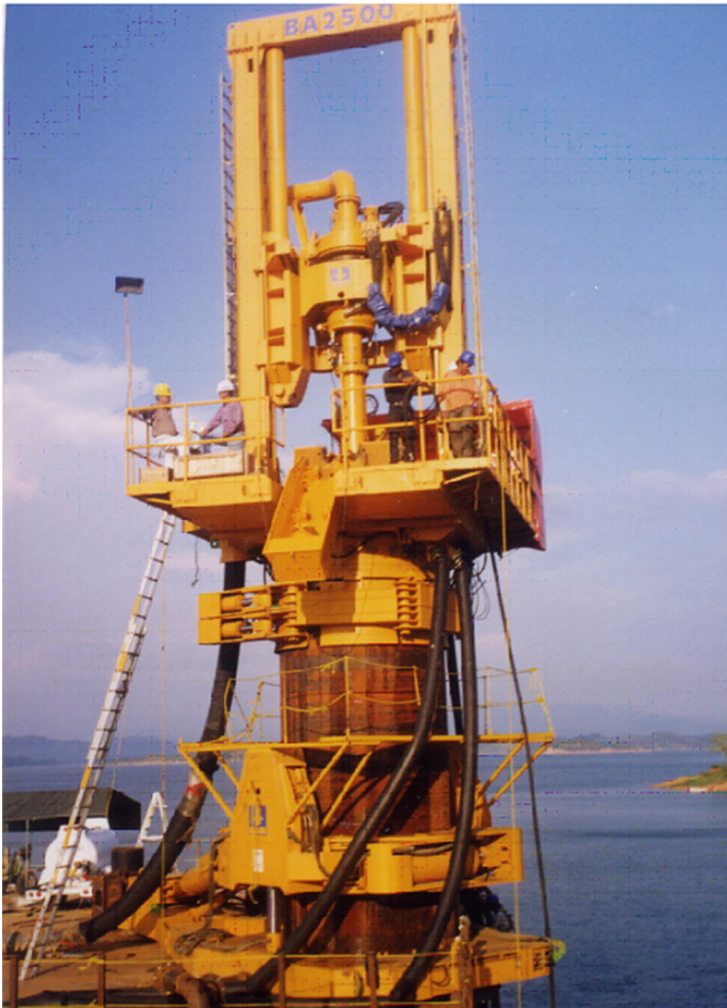
Fig. 1. Top drilling RC unit BA2500 used for installing offshore piles of the Chiapas Bridge in Mexico.
