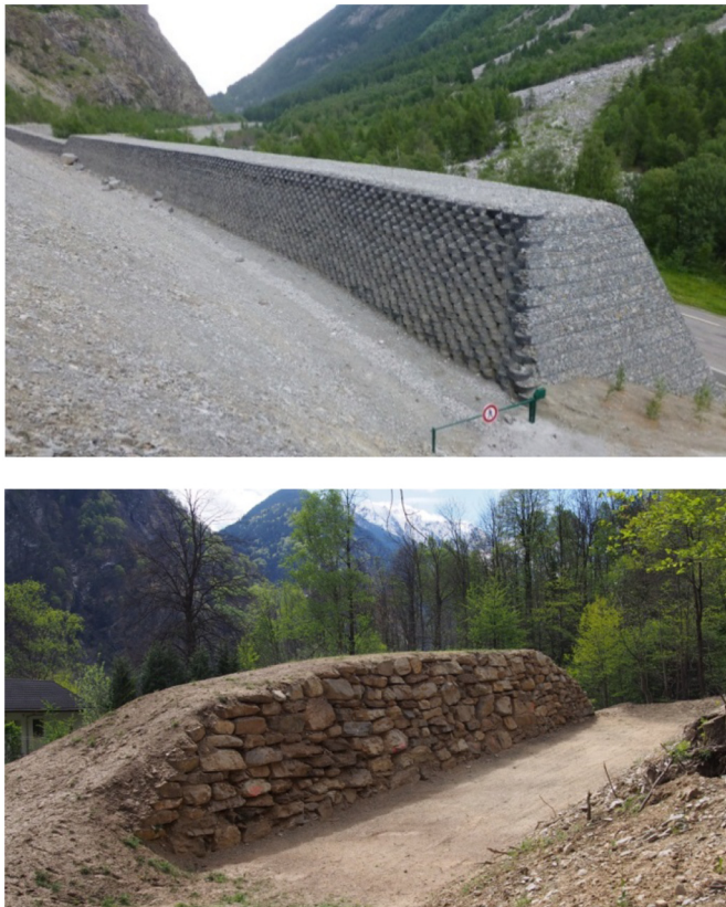
Fig. 1. Example of a 7 m-tall reinforced embankment protecting a road (La Grave, France) and of a small rockery-facing embankment protecting a house (Soazza, Switzerland) (pictures: S. Lambert).
