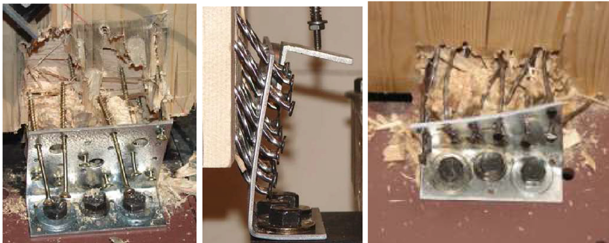
Fig. 1. Damages of traditional non-resilient connectors under reverse cyclic loads: brittle wood failure (a); nails yielding (b), and bracket connector yielding [17] (reprinted with permission).
