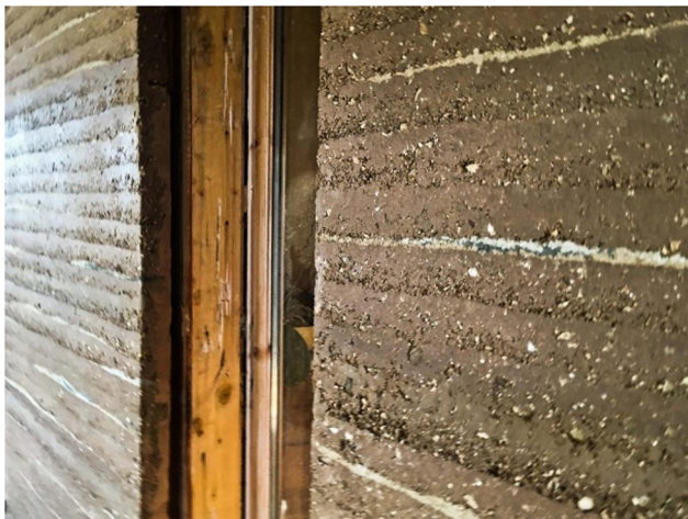
Fig. 1. Example of a RE wall using thin lime layers in France. Source: TERA.
