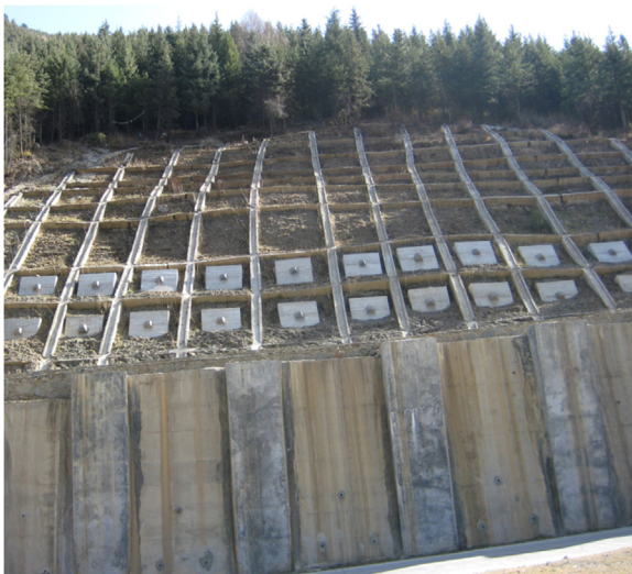
Fig. 1. A sheet-pile wall combined with anchoring frame beam performed well in 2008 Wenchuan great earthquake.
