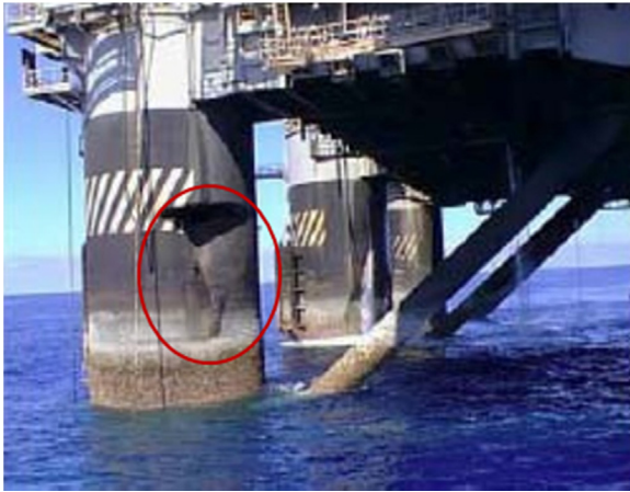
Fig. 1. Damaged platform column [3].
