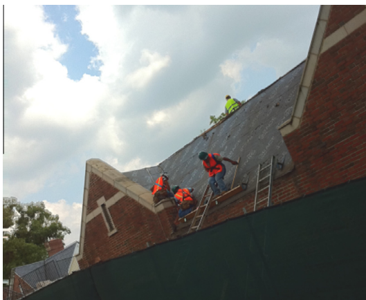
Fig. 1. Worker exposure to safety hazards.
