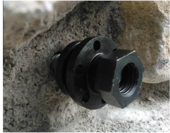
Fig. 1. Cord locking device inside the wall joint before application of steel cords and mortar.
