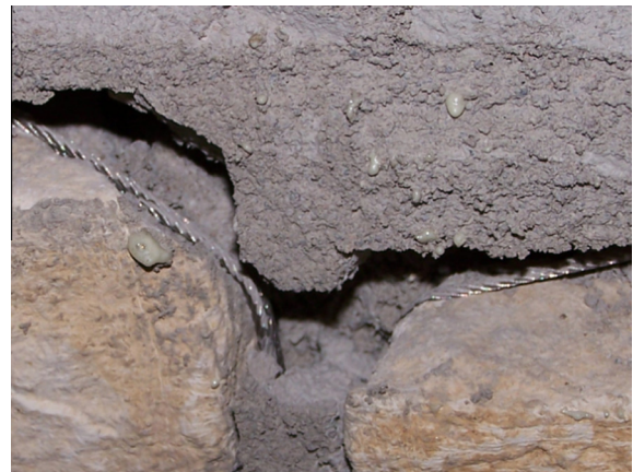
Fig. 2. Stainless steel cord inside cracked (opened) three leaf masonry wall joint under bending load, during failure.
