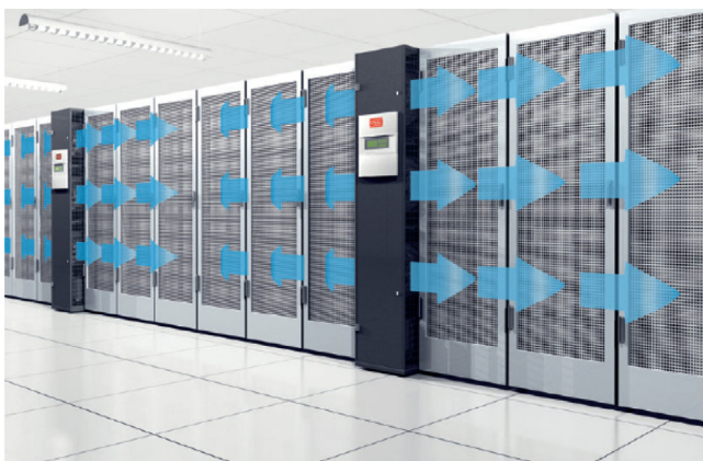
Fig. 2. An In-row air conditioning system in data center.
