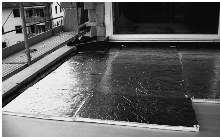
Fig. 2. VIP insulation of a terrace with heated rooms beneath. The panels are placed on a thin polystyrene foam layer for mechanical protection.
