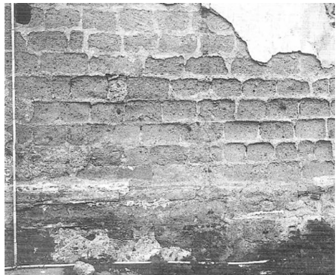
Fig. 2. Bozzette masonry wall (West front wall of the Royal Palace in Portici).
