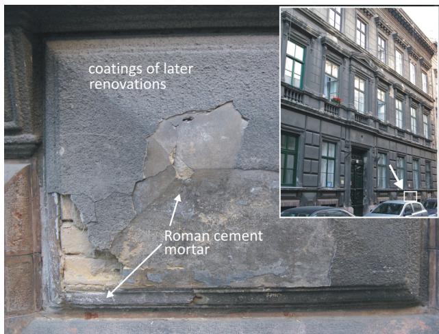
Fig. 1. Characteristic apartment house in the Budapest downtown with slightly damaged diamond-pointed rustication at the plinth made of Roman cement (RC-2).
