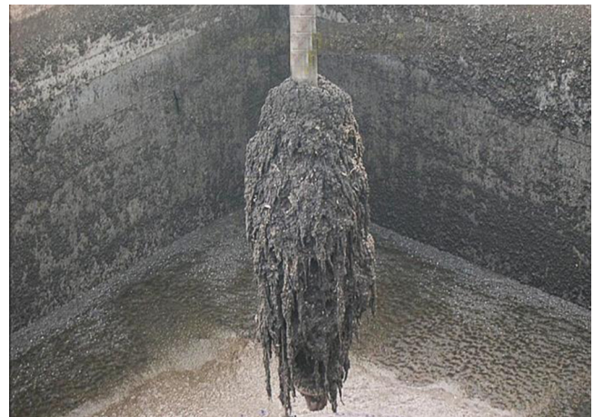
Fig. 1 – Rag accumulation on an impeller lacking anti-rag design properties.
