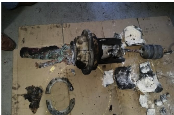
Fig. 1. Broken parts of B-phase HV cable termination and bushing.
