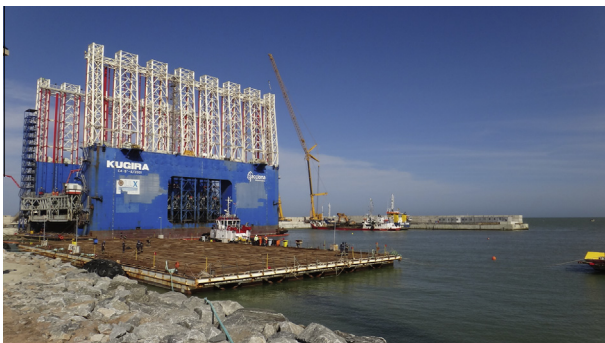
Fig. 1. Construction of breakwaters for a shipyard in São João da Barra, in Brazil.
