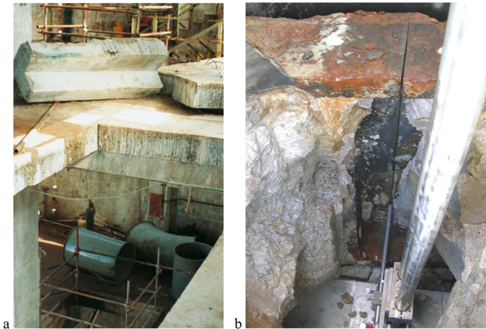
Fig. 1. Cutting of composite structures with hydro-abrasive cutting tools. (a) Cutting of steel bar reinforced concrete members with an abrasive injection tool (Reference: WOMA GmbH, Duisburg, Germany). (b) Cutting of a steel plate covered cementitious composite with an abrasive injection tool (Reference: BHR Group, Cranfield, UK).
