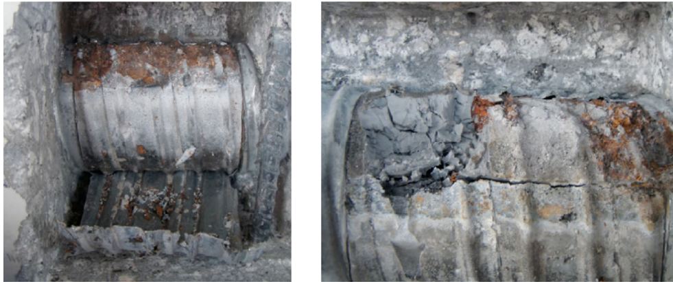
Fig. 1. Duct corrosion and the residual grout in PSC member [12].
