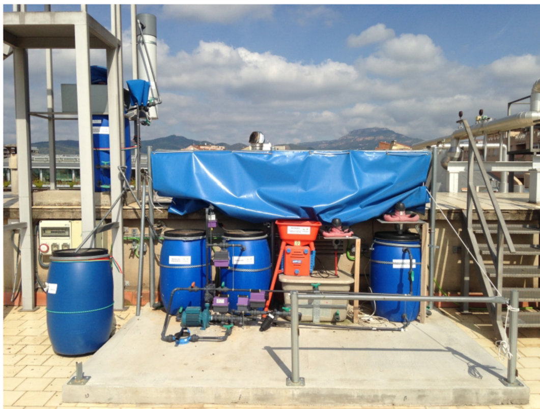
Fig. 1. Prototype of the water purification plant.
