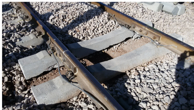
Fig. 1. Signaling gap in Tehran-Karaj railway.
